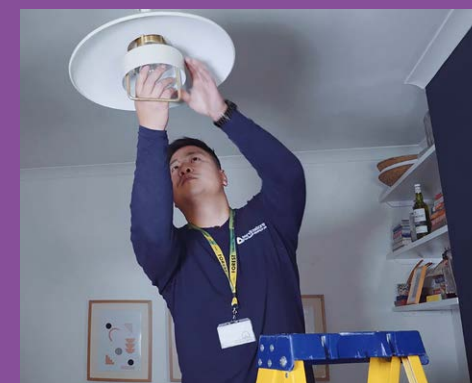
Figure 29: Domestic and communal electrical works
