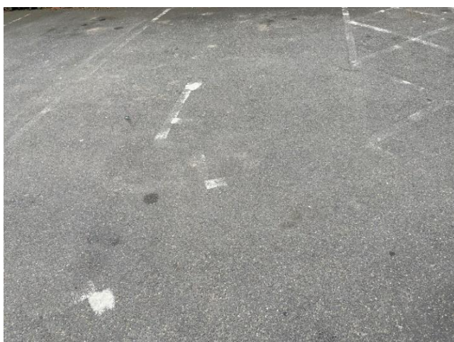
Figure 18 - Worn baylining (New Street)
