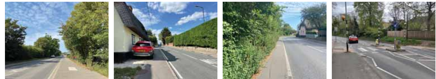
Figure 6.2 Major walking and cycling route along B1256 connecting the west and the town centre(left); Footway parking compromises the footway width; Under-maintained footway with overgrown vegetation and cracked surface; Example of controlled crossing to address severance(right)
