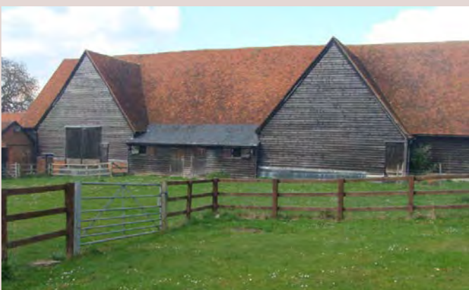
▲ Grade II listed Bury Farm Barn, Felsted, with a restored weatherboarded timber framed and Queen post roof structure.
