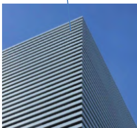
Louvres to external plant enclosure
