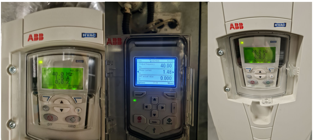
Figure 3: Multiple AHU VSD readouts
