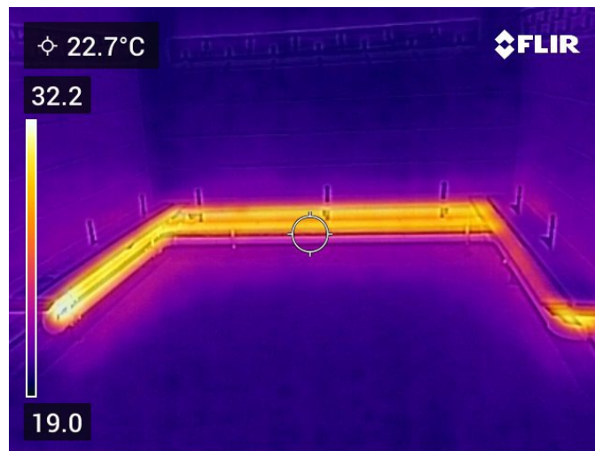
Figure 15: Under bench heating in sports changing rooms left on when not in use
