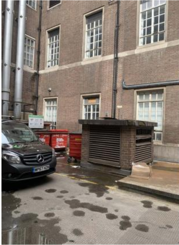
• Courtyard with plant equipment, vents from basement & parking
