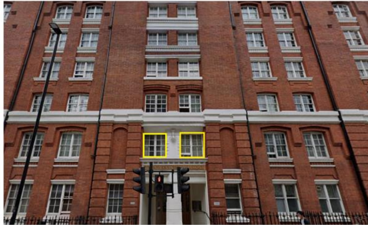
Figure 05: Windows falling below guidance for AP SH outlined in yellow (Queen Alexandra Mansions)
