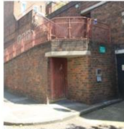
3. Proposed heating pipes to come up through floor of existing plant room located underneath external ramp at Alexandra Place
