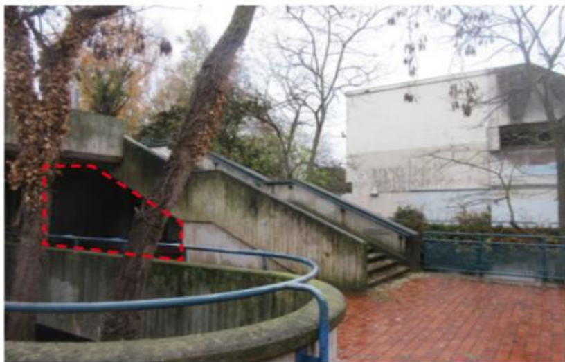
View of enclosure area below the stair. Proposed Sub-Plant Room highlighted by red dotted line
