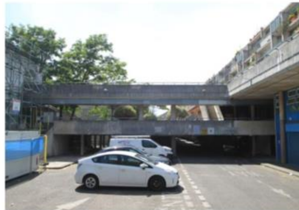
View from level 02 of car park entrance showing existing high level route to Block A. Casing to be replaced by smaller/higher pipework
