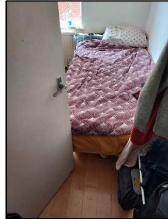
Bedroom of 5.6m 2 , below national statutory minimum, being let
