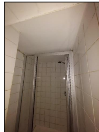
Cause investigated and replastered
