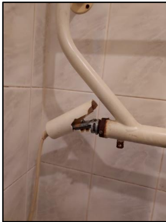
Exposed electrical component presenting risk of electrocution
