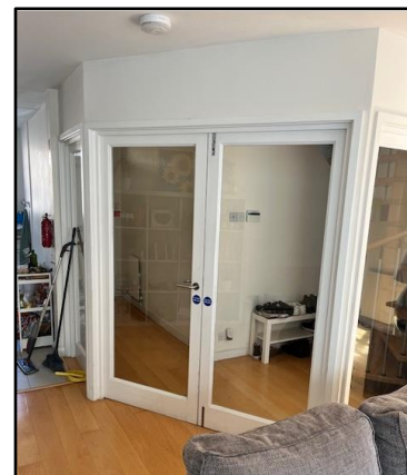
This work physically separated the means of escape thereby improving fire safety
