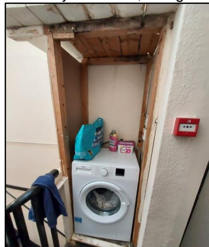
Washing machine in means of escape
