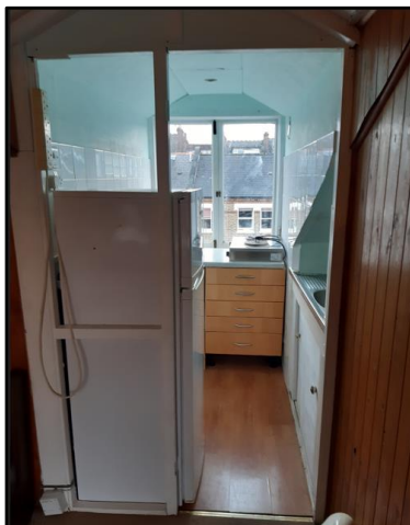
Fire safety issue from lack of door and partition to separate the kitchen from means of escape
