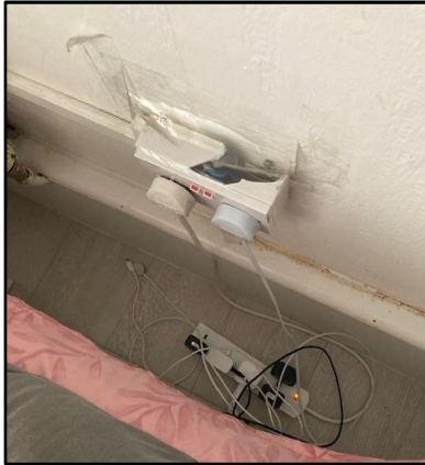
Broken electrical sockets with exposed wiring
