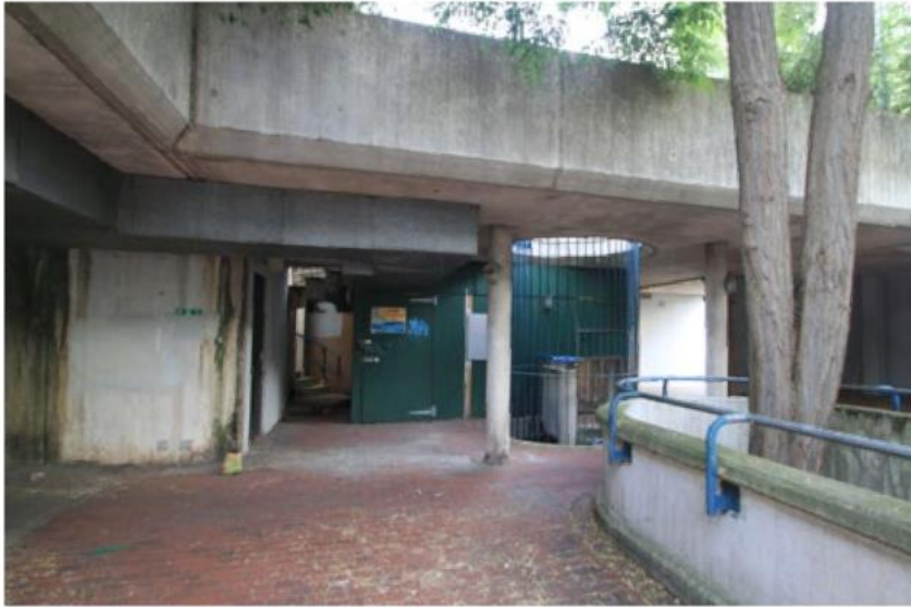
Existing ductwork fixed to soffit of walkway, connecting boiler room to block A5
