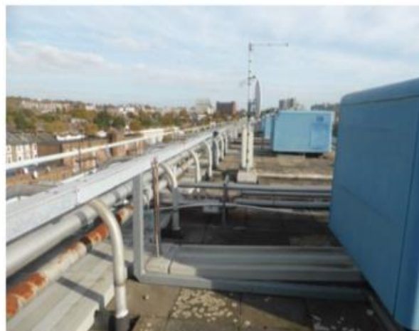
Image 2: Existing heating network on roof of Block A
