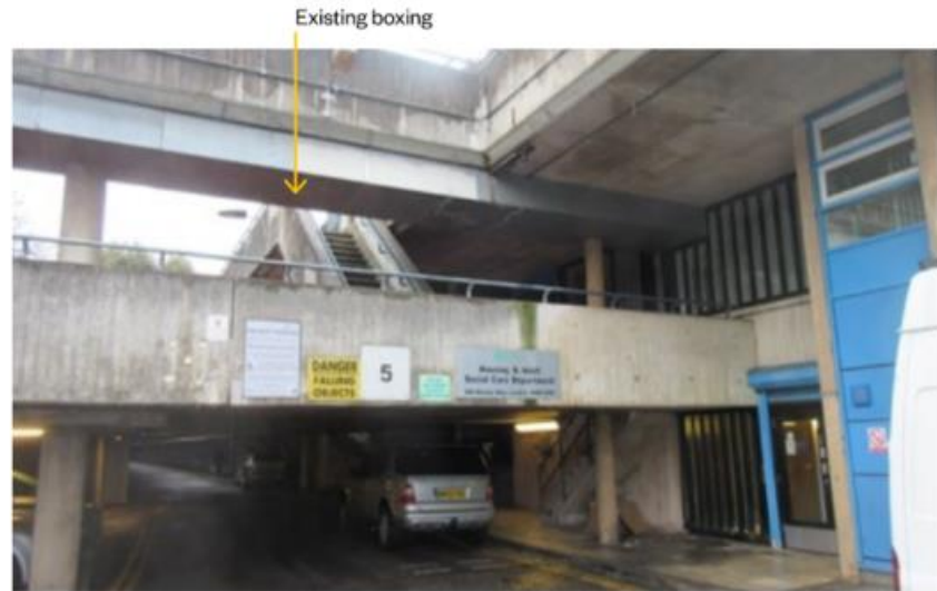
Existing condition of boxed section fixed to walkway soffit and penetration point to Housing Office fenestration
