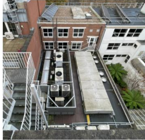
Plant equipment on 'link' structure roof
