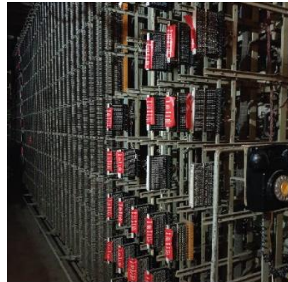
4 Main Distribution Frame
