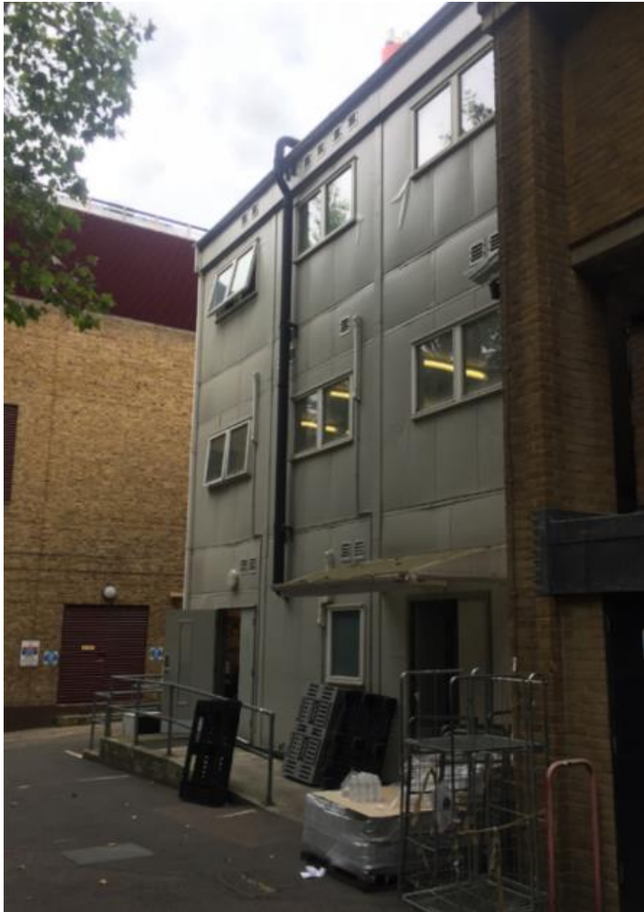
Figure 2 – The existing SW Portacabins that provides welfare facilities for the contractors who work at the Museum.
